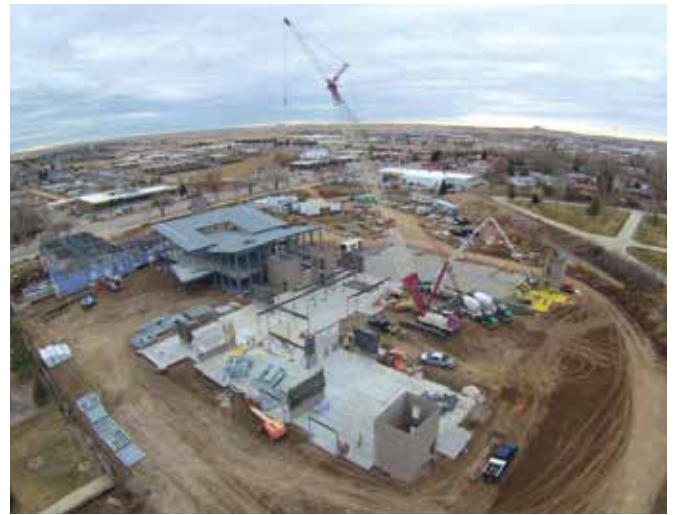
Aerial photograph of The Legacy Living and Rehabilitation Center. Courtesy of J. Scull Construction.
